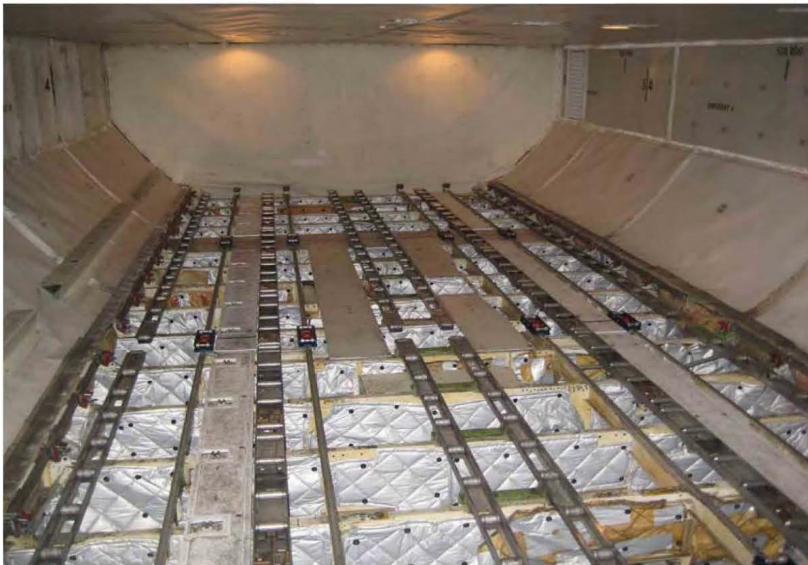
Lower Deck Cargo Loading System
