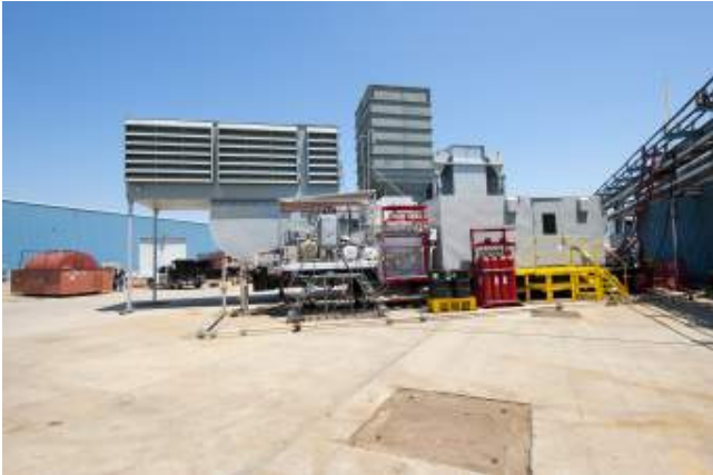
Control Room Side
