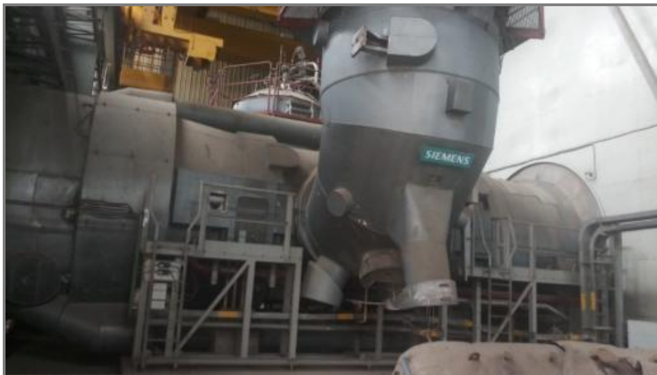
Gas Turbine GT# 1B
