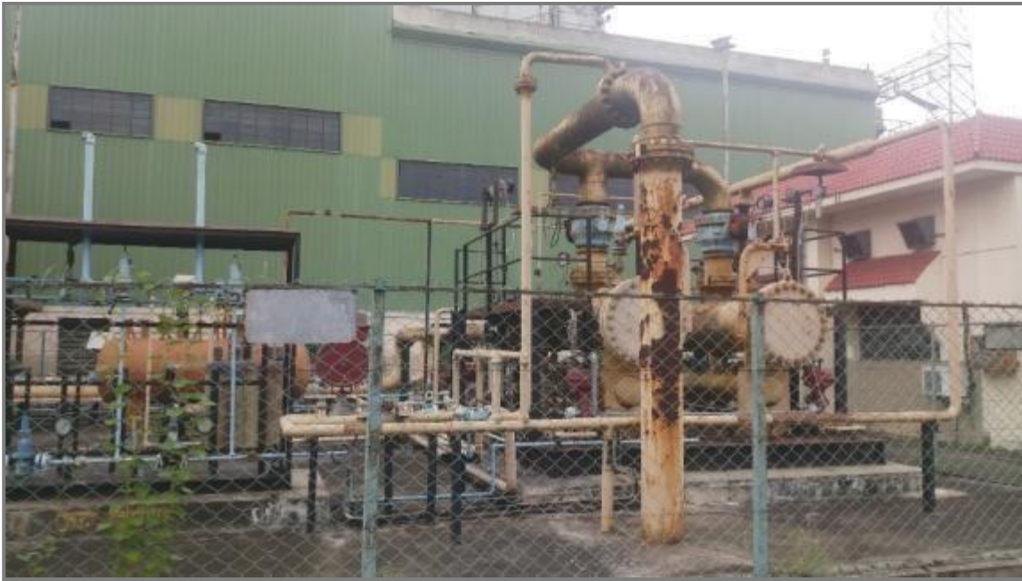
Gas Conditioning Skid
