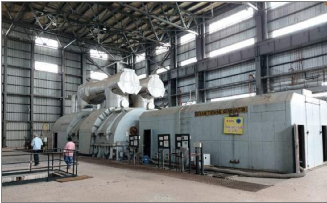
Steam Turbine & Generator
