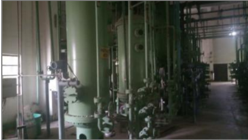
DM Water Plant
