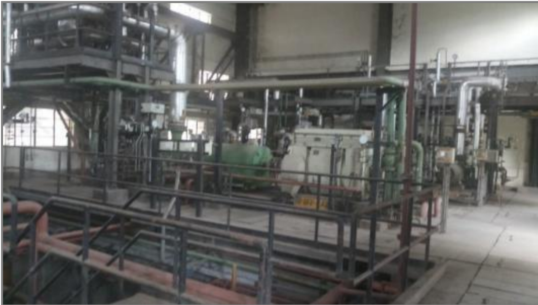
Steam Turbine Auxiliaries
