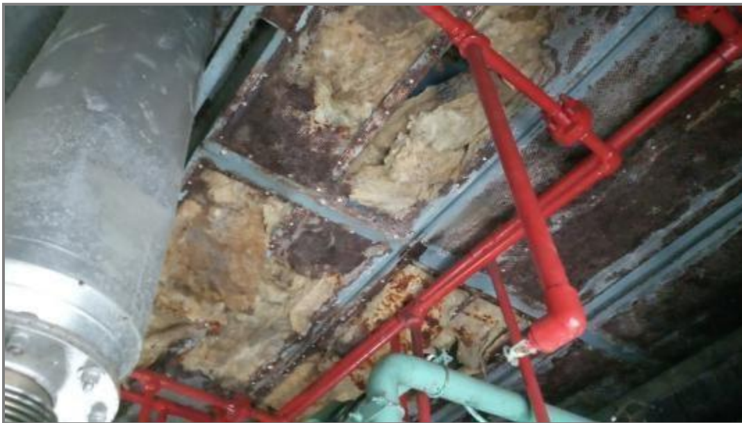
Top enclosure of DG Set
