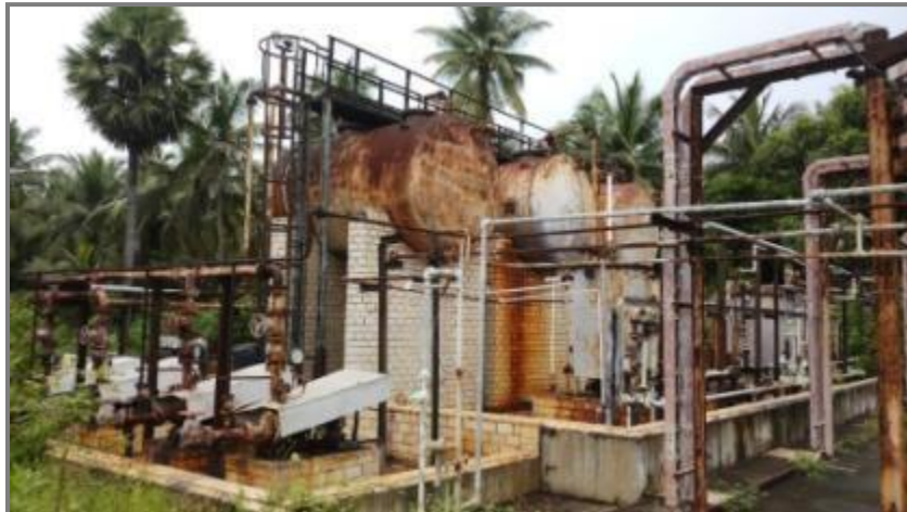
tanks for DM plant
