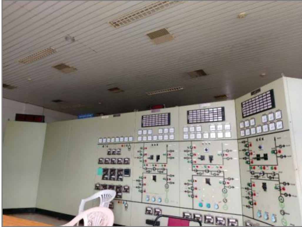
Switch yard Control
