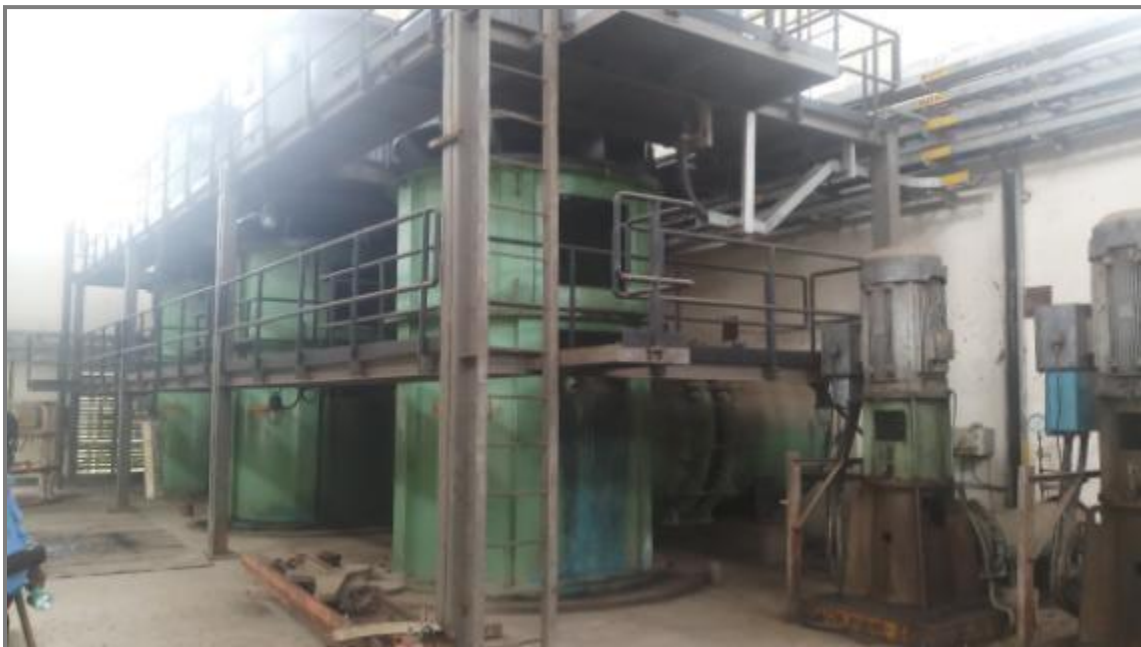
Cooling Water Pumps
