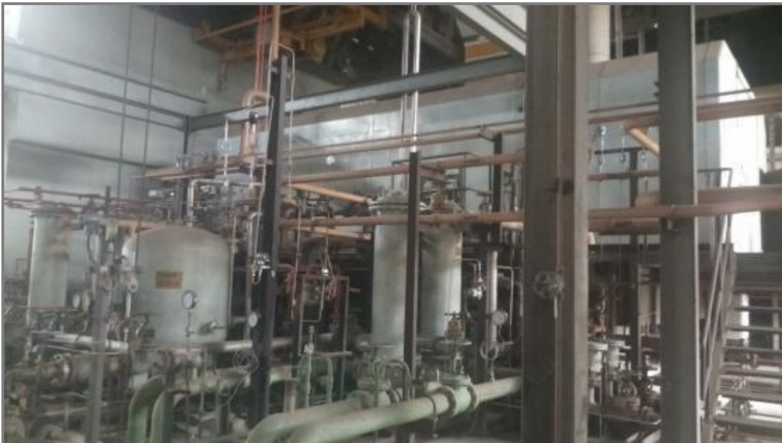
Gas Turbine Generator & Auxiliaries
