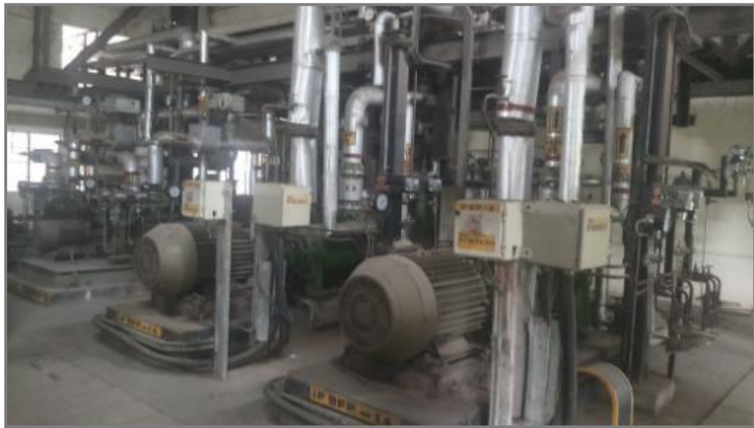
Condition of IP Boiler Feed Pumps
