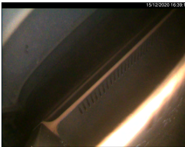
Picture 29: stage 2 nozzles
