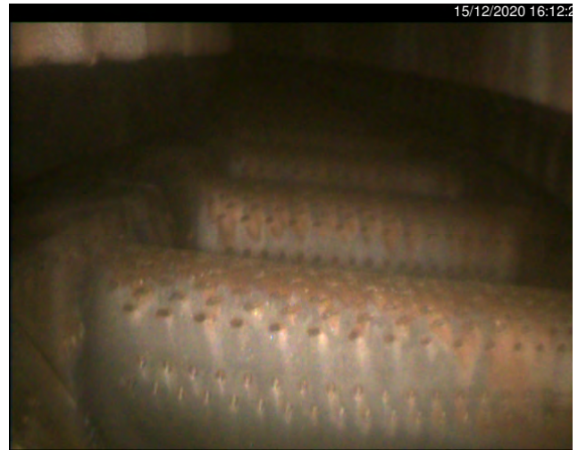
Picture 20: stage 1 nozzles
