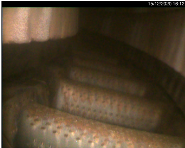
Picture 19: stage 1 nozzles
