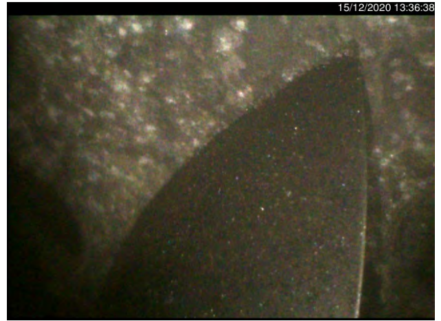
Picture 8: salts and deposits
