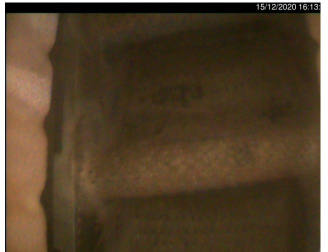
Picture 22: stage 1 nozzles
