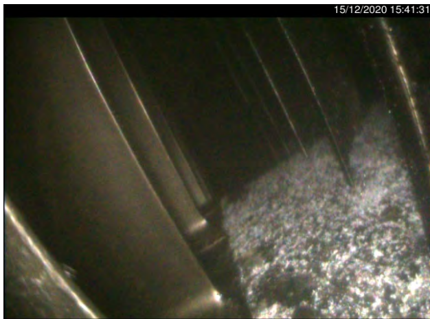
Picture 9: salts and deposits
