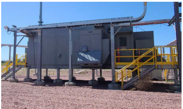
6500 HP VFD E-HOUSE
